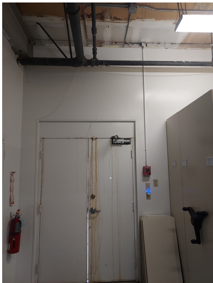
Archive with water damage and gaps to exterior in door.
